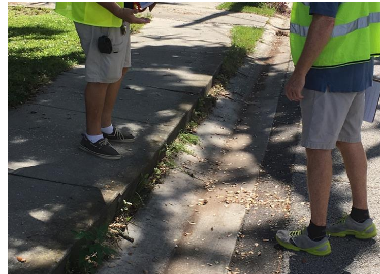
Vertical separation of sidewalk panel along 7 th Ave. N.
