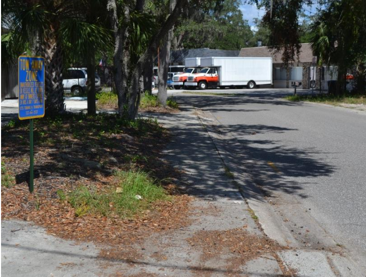
Poorly maintained sidewalk along 10 th Ave. S.
