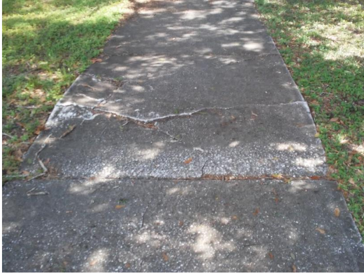
Deteriorating sidewalk along Marshall St.
