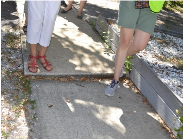
Vertical separation of sidewalk panels along SR 590
