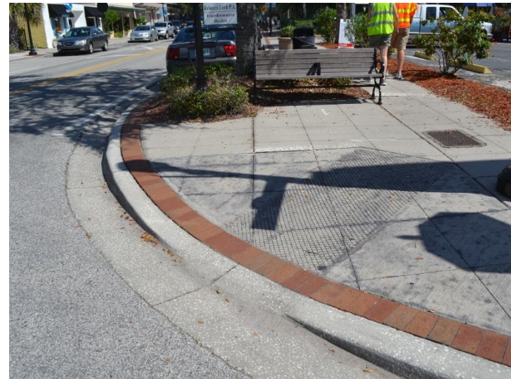
Poorly designed ADA curb ramp along Main St.
