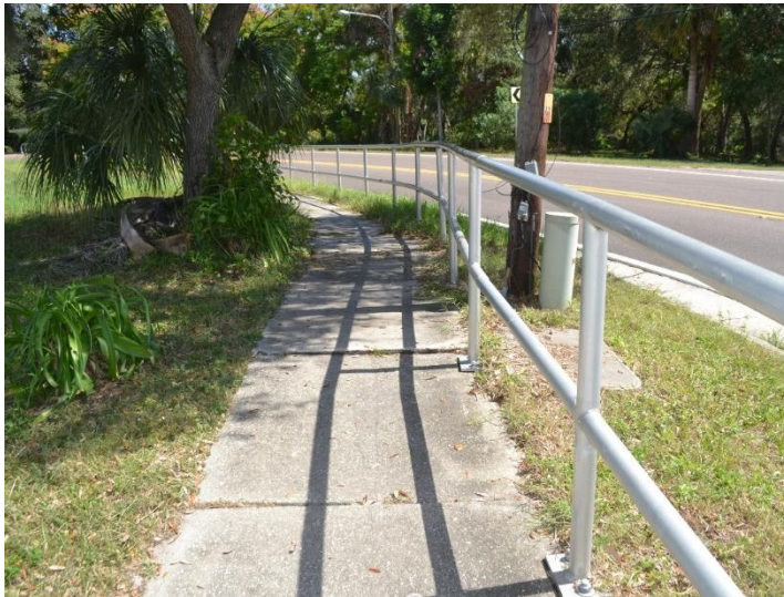
Vertical separation of sidewalk panels along SR 590
