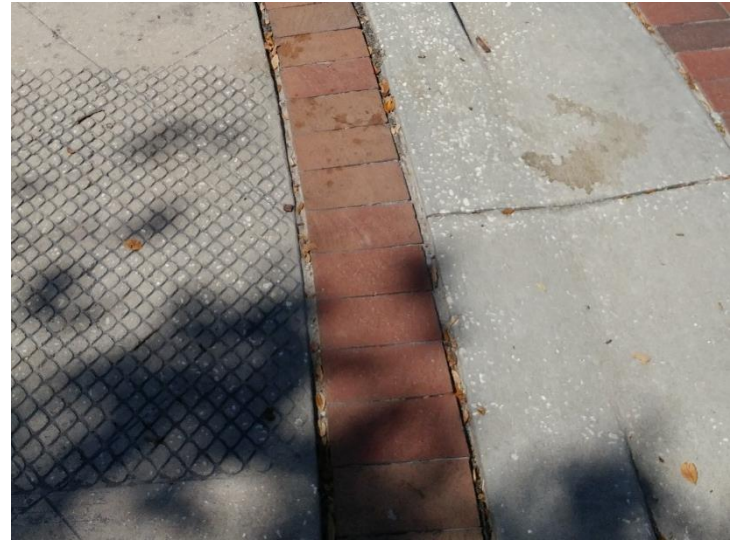
ADA curb ramp lacking truncated domes on Main St.
