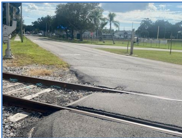
Sidewalk gap at CSX tracks
