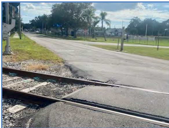
Sidewalk gap at CSX tracks
