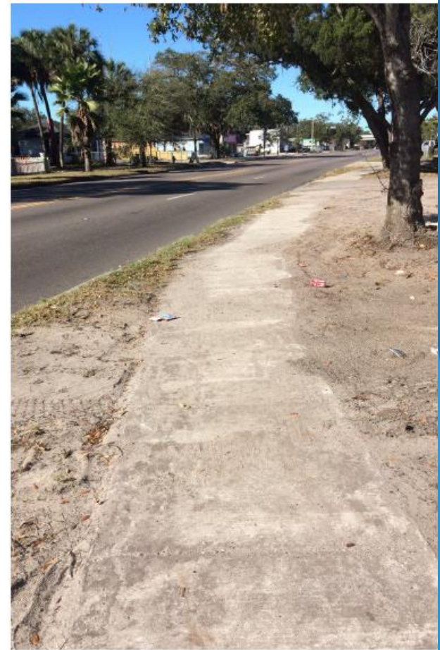
A sidewalk in need of repair on 18 th Avenue South.
